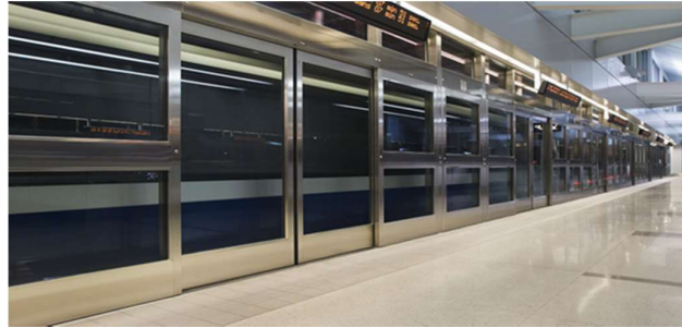
Fig. 3. Sliding doors on a station
